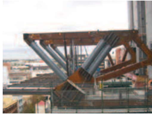
The success of the Latitude@ World Square construction process hinges on these huge "jump start" trusses, effective in large part due to the light weight and great strength of Bisplate 80.
